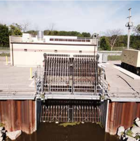
New self-cleaning trash rack.
