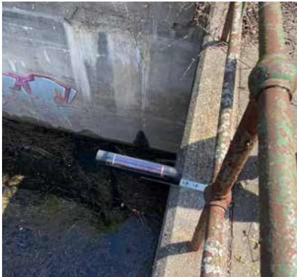
Debris detection at Beyer Dam in Washtenaw County
