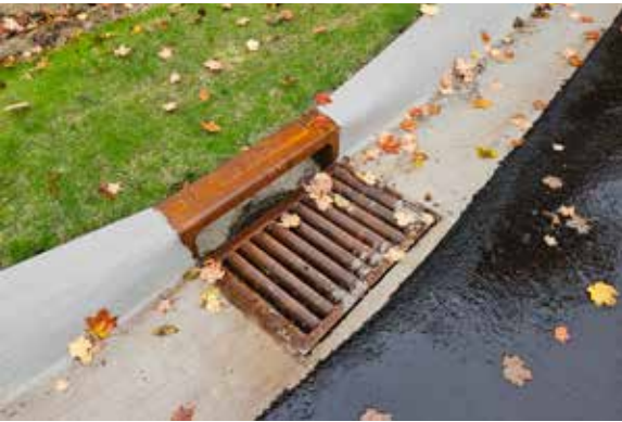
A high-flow capacity catch basin
