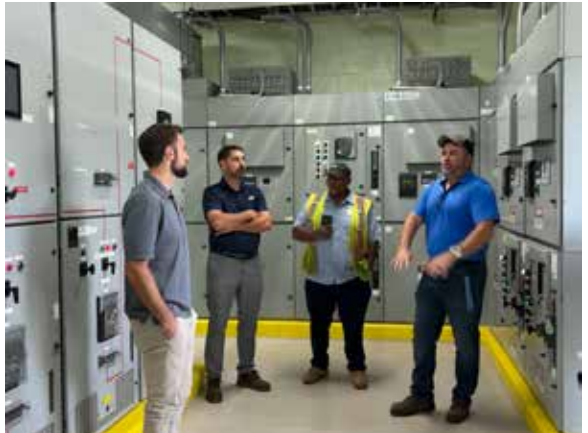
Officials receive an explanation of electrical system upgrades to improve reliability and efficiency of Milk River facilities.
