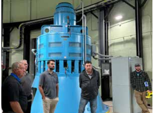
State and local officials get a close-up view of refurbished storm pumps at the Milk River Intercounty Drain CSO RTB.
