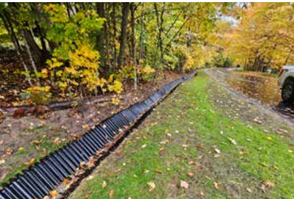
One of the "Smart Ditch" products used during the project
