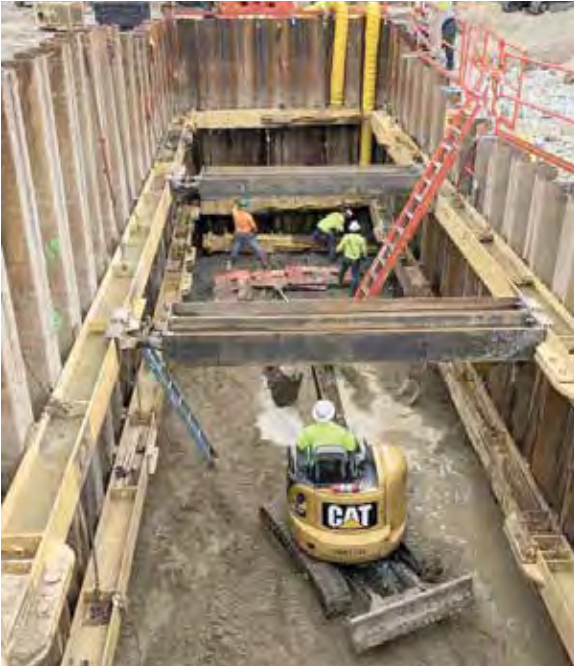
It was determined that an approximately 32-foot-long section of the sewer would need to be excavated and replaced. The ground water table within an upper aquifer was lowered approximately 20-feet and a sheet pile access shaft was used to support the excavation.
