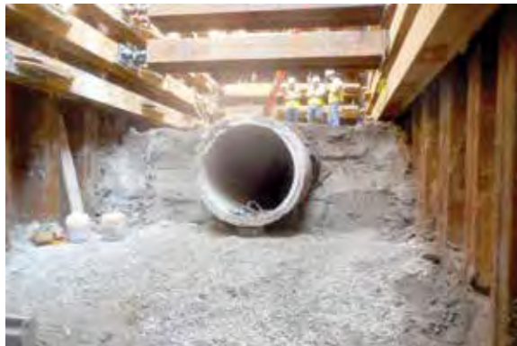
Using a modular shoring system to expedite access shaft excavation, a 37-foot-deep excavation was needed to expose and replace the section of damaged 54-inch diameter sewer.
