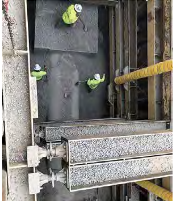
Thirty-two feet of 54-inch diameter pipe was replaced. Heavily reinforced collars at the ends were designed to ensure a worry-free connection between the existing sewer pipe and the replacement pipe.
