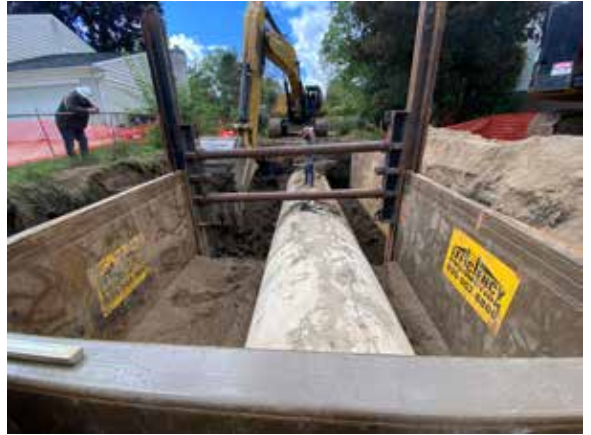
Removal of existing 66" storm sewer for the installation of the outlet control structure.
