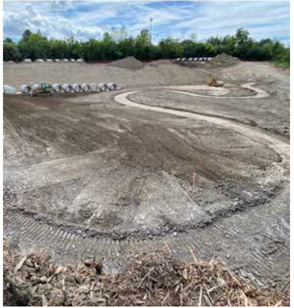
Rough grading of the low flow channel in the bottom of the floodplain area.
