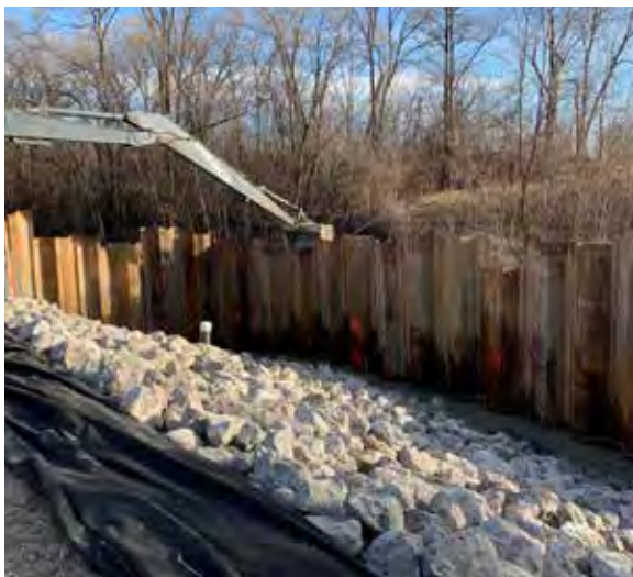
Booms placed on the Bear Creek in Warren and the first of the steel sheeting to isolate the contaminated area to begin remediation, after a Macomb County Public Works inspector noticed old diesel fuel in the water.
