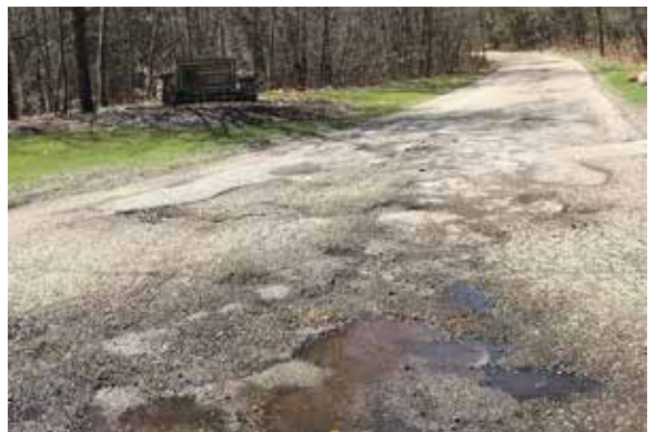
Repairs to the long crumbling roadways within the park were the focus of the DNR's multi-phased ARPA-funded project that took place concurrently with the drain project.
