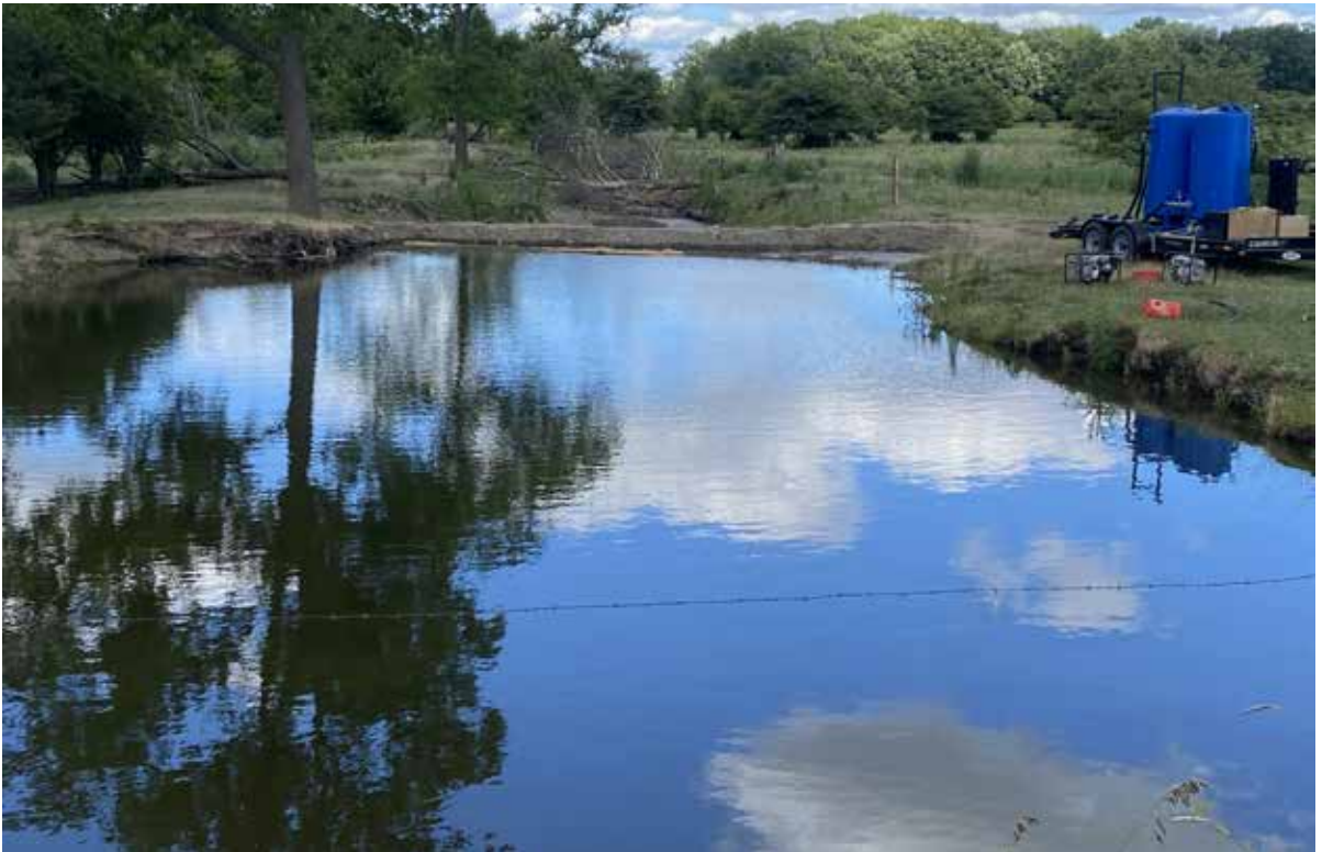
Mobile filtration system set up at downstream dam to clean flow affected by initial spill plume. Filtered water was discharged downstream.
