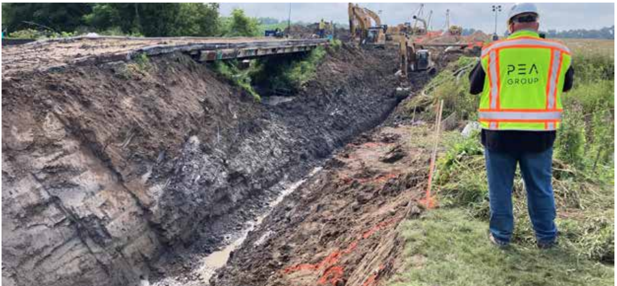
Open cut through Dietz Creek Drain approximately 25 feet deep to install 36-inch gas pipeline.
