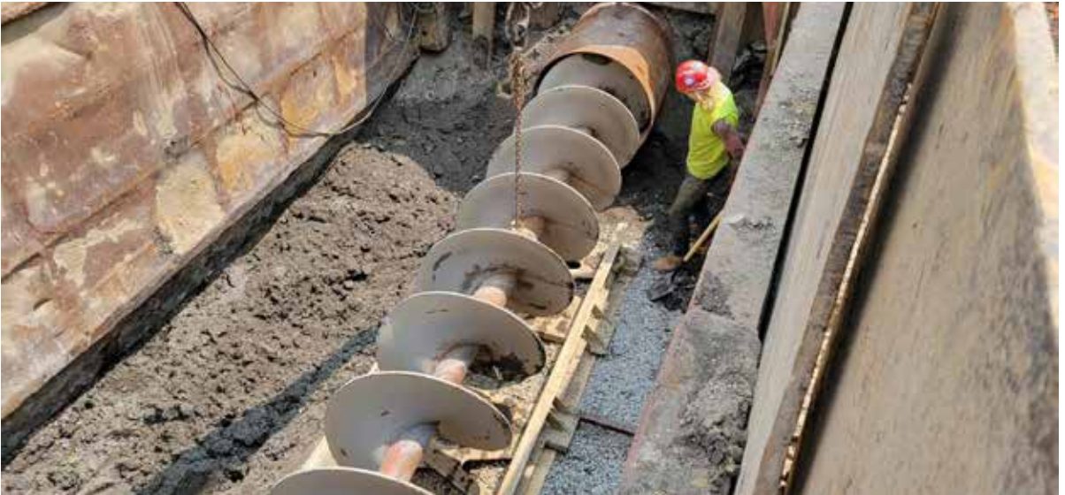
Jack & Bore crossing of the Locke Drain, City of Perry, Shiawassee County.
