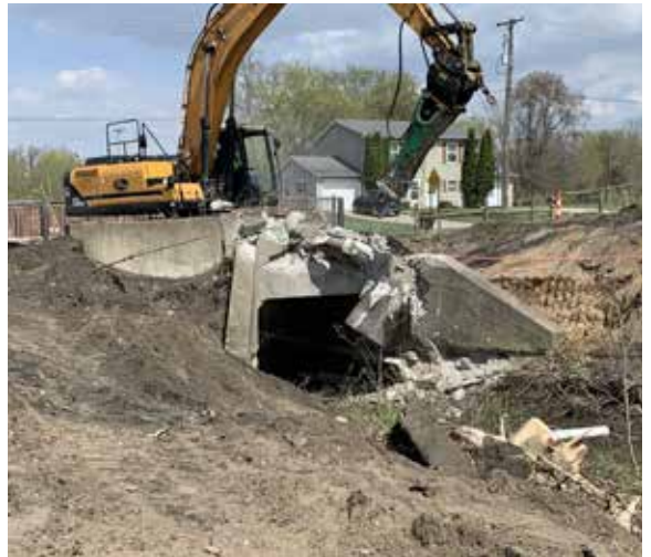
Demolition of the Great Lakes Central Railroad Crossing on the Little Tobacco River Intercounty Drain.
