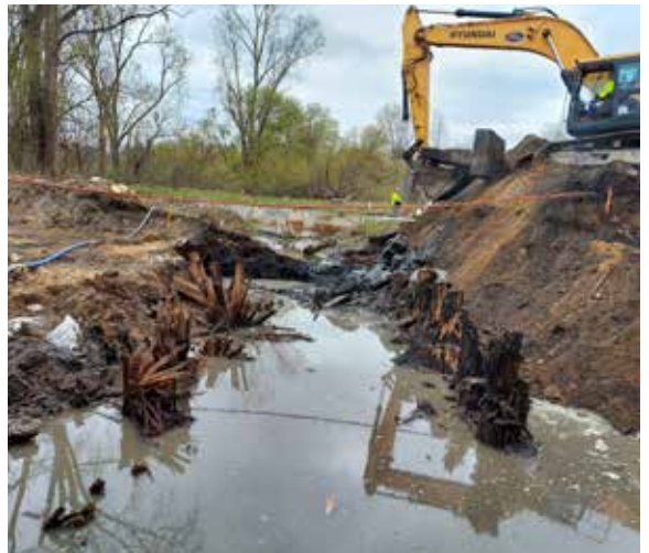
Demolition of the Great Lakes Central Railroad Crossing along the Little Tobacco River Intercounty Drain in the City of Clare.
