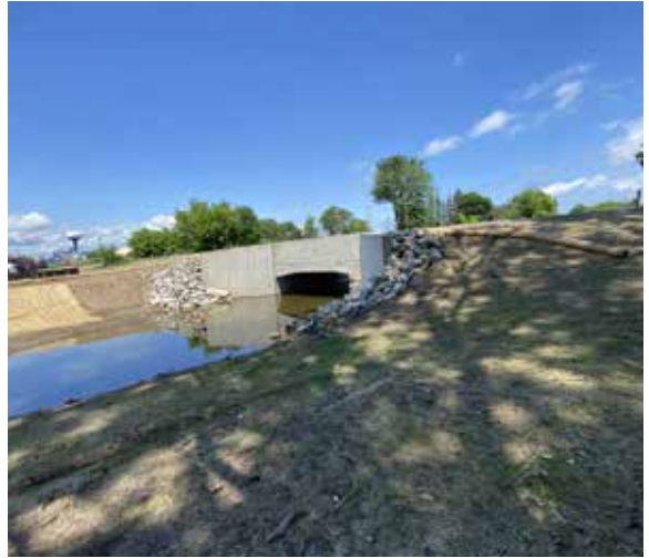
Demolition of the Great Lakes Central Railroad Crossing along the Little Tobacco River Intercounty Drain in the City of Clare.
