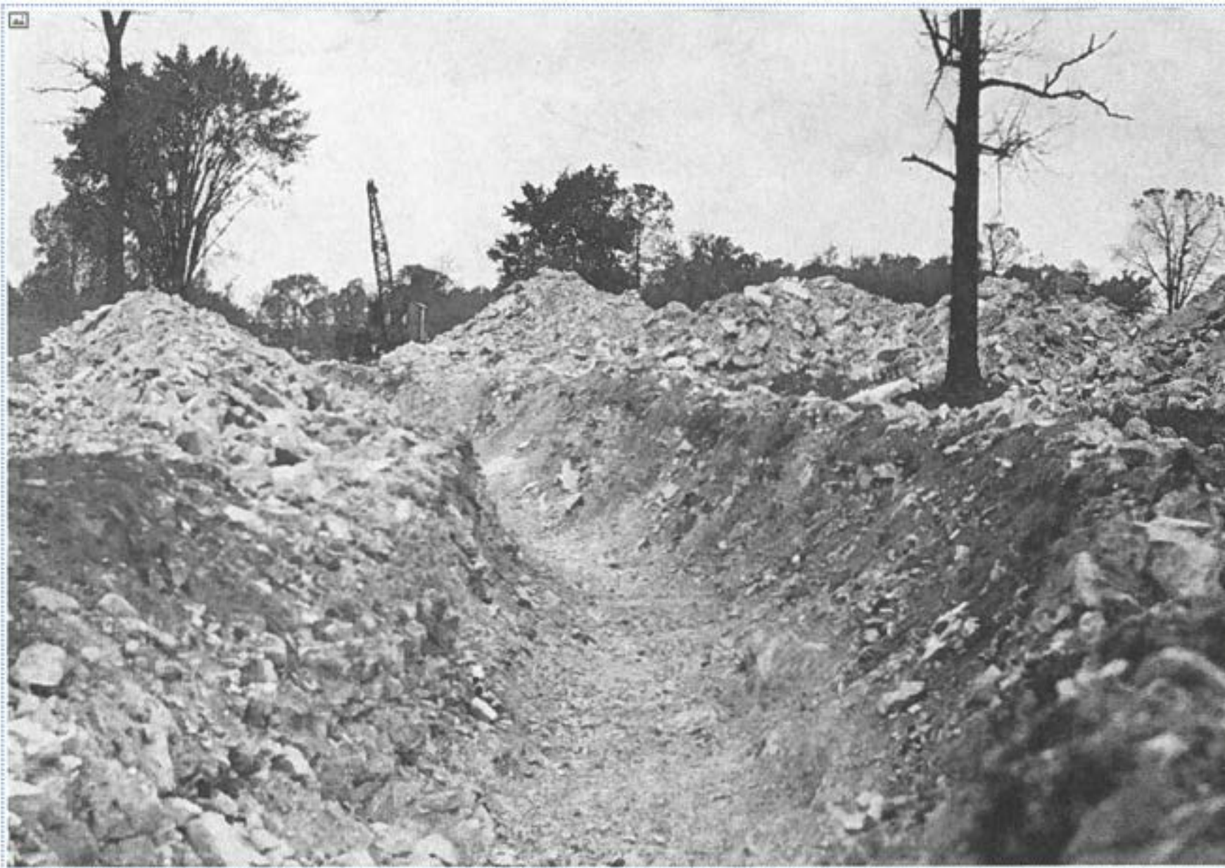
Inter County Drainage Construction. Hills do not interfere or have any barriers between marshes. Modern equipment comes straight through.
