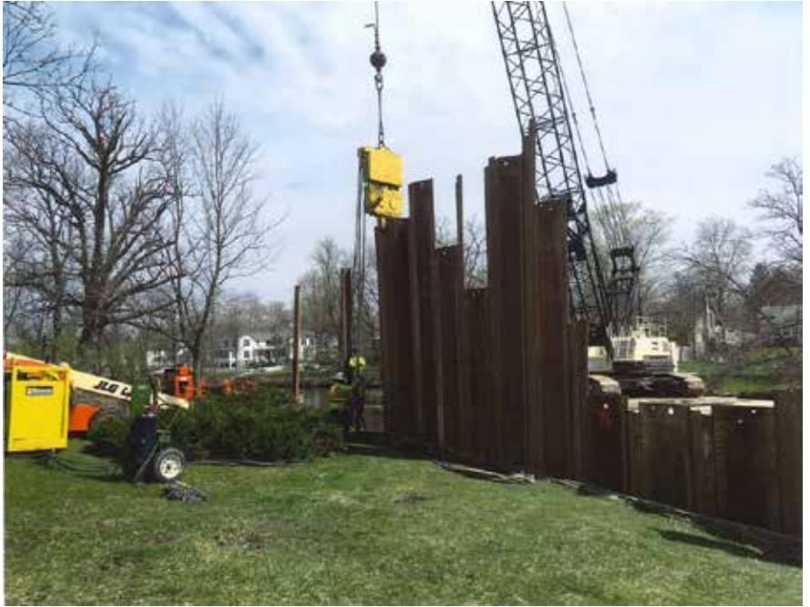
The rehabilitated southeast, northeast, and northwest quadrants of seawall include steel sheet piling and concrete caps.
