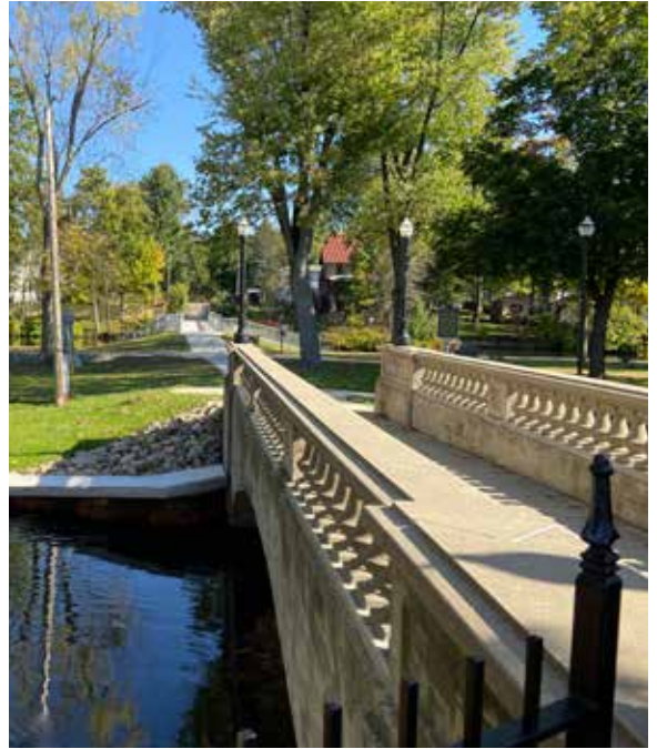
This project brought G.A.R. Island Park into ADA compliance by lowering the deck bridge.
