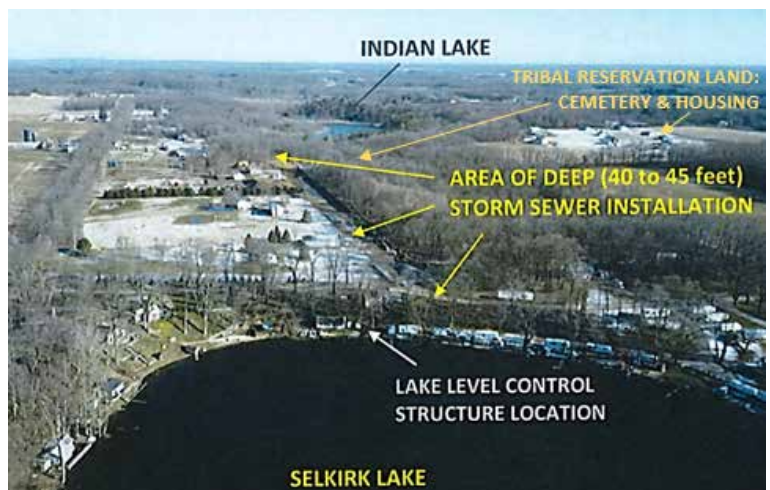
This drone photo, taken during construction in 2017, shows the various aspects of work relative to the two lakes and the tribal owned properties.
