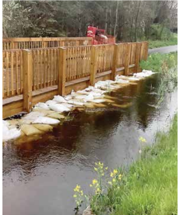
Looking North at the Beechtree Drain along 168th Ave. in Grand Haven Township after the historic May 2020 storms. The OCWRC used diesel pumps and sandbags along the drain to mitigate flooding.
