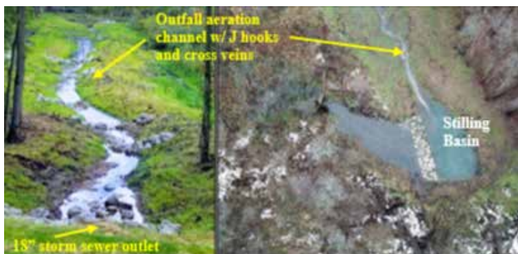
A 550 ft. long outfall aeration channel (picture top left, looking north), with J hooks and cross vanes, constructed to help increase the oxygen levels by aerating the discharge water, spills out into a stilling basin (picture on the right, looking southwest). Once that overflows, the runoff uniformly discharges through the emergent wetland, through no discernable path, until it reaches Indian Lake approximately 700 ft. away
