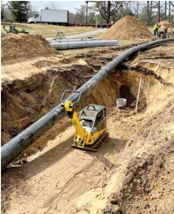
Storm sewer pipe about to be directionally drilled under Retreat Dr. adjacent to American Dunes Golf Course. This new infrastructure connected previously separated portions of the Beechtree Drain.
