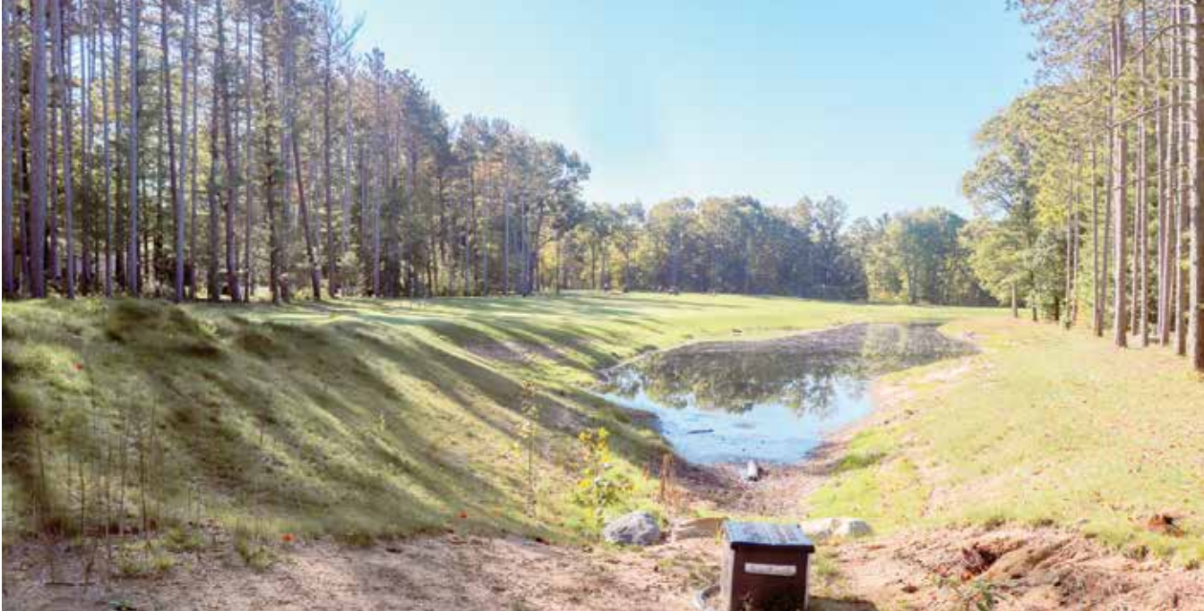
Water level control structures were installed as a part of the Beechtree Drain Improvement Project to allow the OCWRC to efficiently control storm water storage and flow along the drain.
