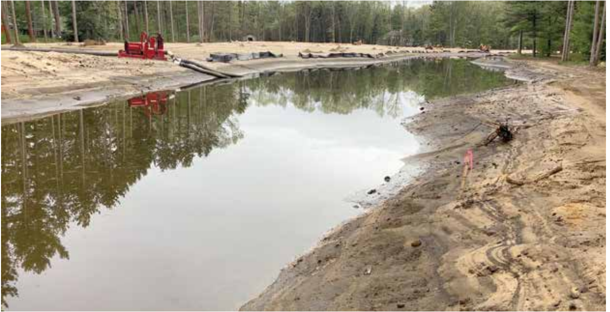
The OCWRC mobilized 4 diesel pumps along the drain to be used prior to and during construction to manage storm water levels within the watershed.
