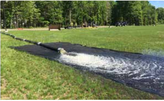
Temporary Pumping Discharge Point at Western Diversified Plastics – May 2018.
