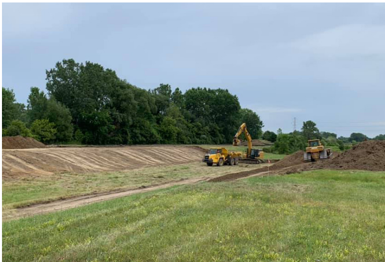
Work is underway on the Sterling Relief Drain in Sterling Heights, Mich. The drain serves roughly the middle third of the city, providing drainage to more than 20,000 residents and hundreds of businesses, including several auto plants and major defense contractors. The underdrain is being daylighted to transform this rather industrial looking drain in something that will be much more esthetically pleasing while continuing to be an effective drain for the community. Major construction will wrap up in late fall, with planting of plants and trees happening by the end of the year or in spring, as weather dictates.
