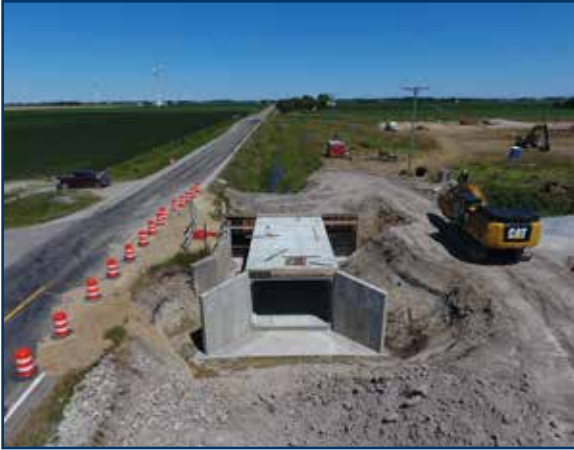
UAV Looking East at view over Quanicassee Road Bridge showing Centerline Drain Project Area
