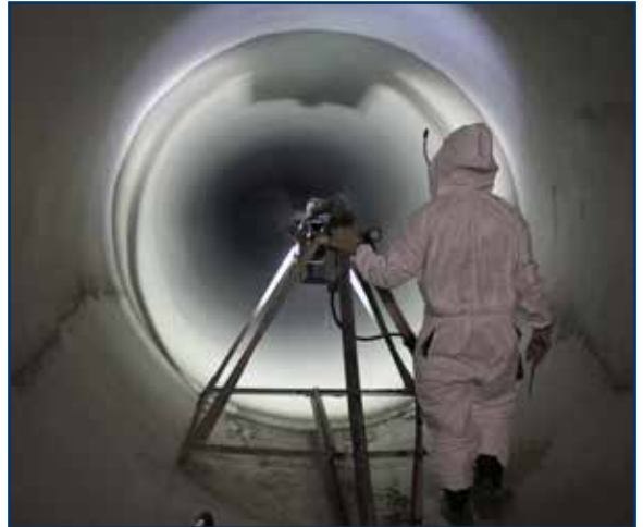
Geopolymers can be centrifugally cast to create a new structural pipe inside of the old pipe.
