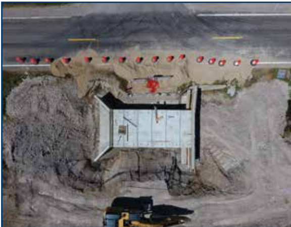
Quanicassee Road Bridge adjacent to M-138 Project from UAV overflight of Centerline Drain
