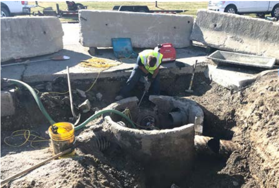
Repair work being conducted at the Murdock-Ballard Pump Station in Harrison Township on Tuesday, July 17.
