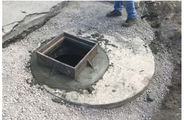
A temporary sewer grate installed on the Murdock-Ballard drain in Harrison Township. The grate will be replaced again in August when final repairs are made on the pump station.
