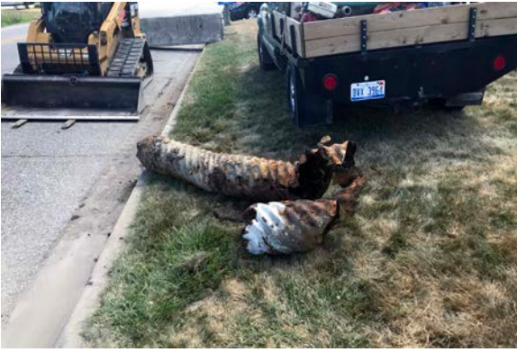
Damaged pipe that was removed from the Murdock-Ballard pump station. The pipe was further damaged during the removal process. A new section of pipe was installed.
