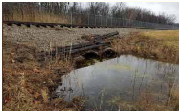
A view of the Gohl drain on the west side of Selfridge Air National Guard Base.
