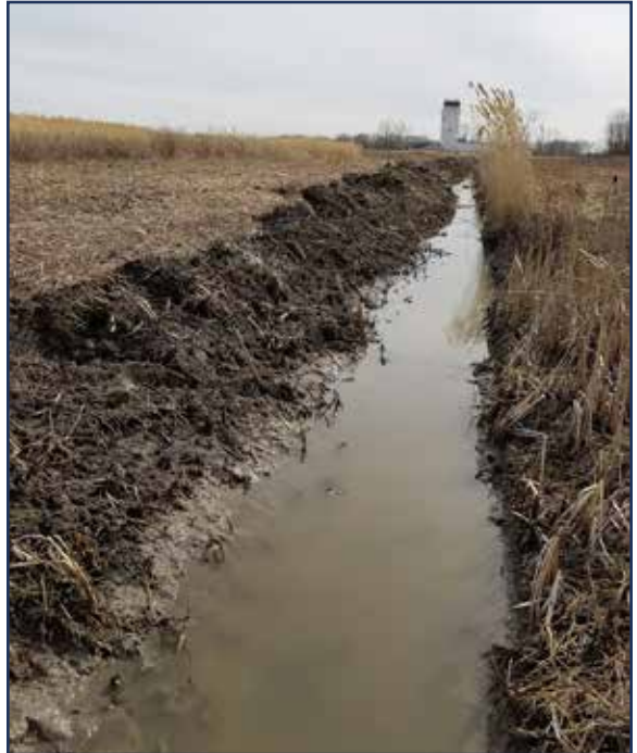
The Air Traffic Control tower at Selfridge Air National Guard Base is seen in the background of this photo of the Irwin Drain.
