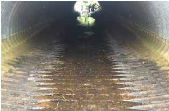
Existing culvert invert with moderate to severe section loss
