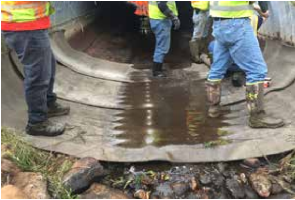
Layout of transverse strips of CC8 fabric at the culvert outlet, shingling in the direction of flow
